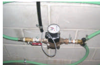
Figure 5: Low Flow Meter
